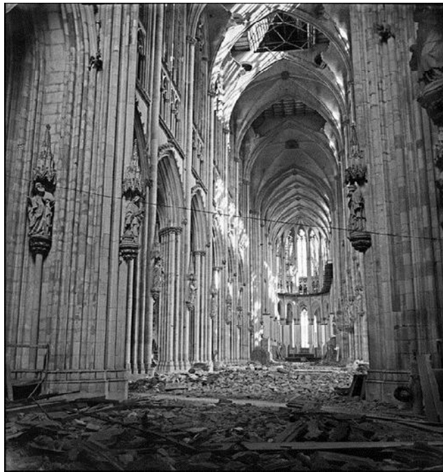
Gambar 1.3 Werner Bischof 1946 Germany Cologne The Interior of a Shattered Cathedral. (Sumber : pinterest.com )
