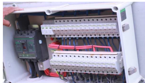
Gambar 8. PVBx (Photovoltaic Combiner Box)
