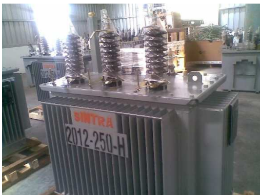
Gambar 1. Transformator Distribusi (Sumber :
