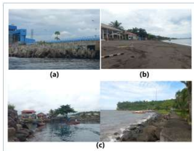
Figure 5. Types of coastal protection structures on the Kema Coast
