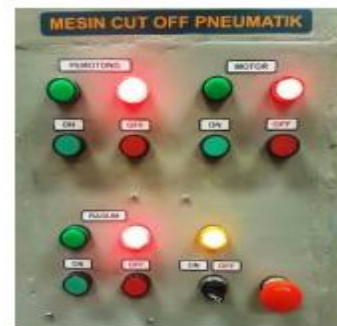
Gambar 4.8 Panel Kontrol Selector Swtch ON
