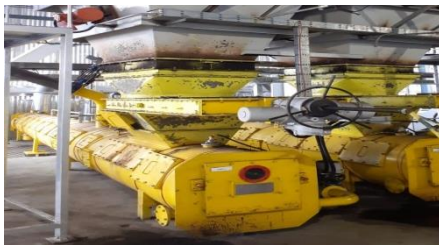
Gambar 2.7 Coal Feeder unit 1 PLTU Sulut-3
